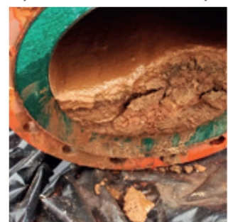
Sludge in pipes
